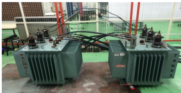
Figure 1. Photo of a distribution transformer with a capacity of 100 kVA
